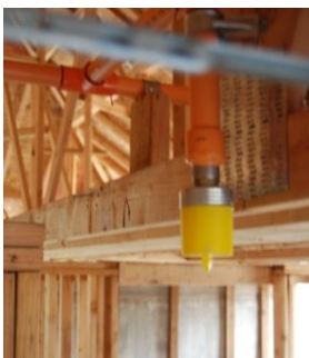
Reliable Automatic Sprinkler Co. donated all of the system components.
