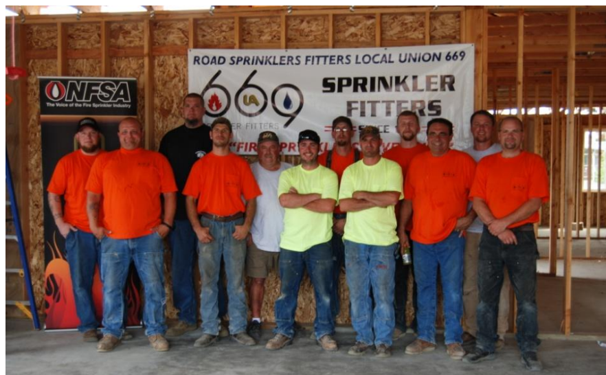
Local Sprinkler Fitter Union 669 volunteers pose for a photo after installing the fire sprinkler system. They look pretty cool despite the 100 degree day!
