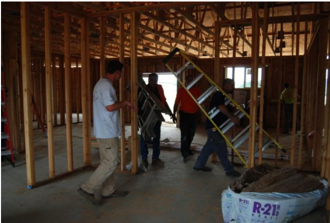
More than a dozen volunteer sprinkler fitters made short work of the system installation.
